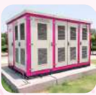
BAJAJ COMPACT SUB STATION
